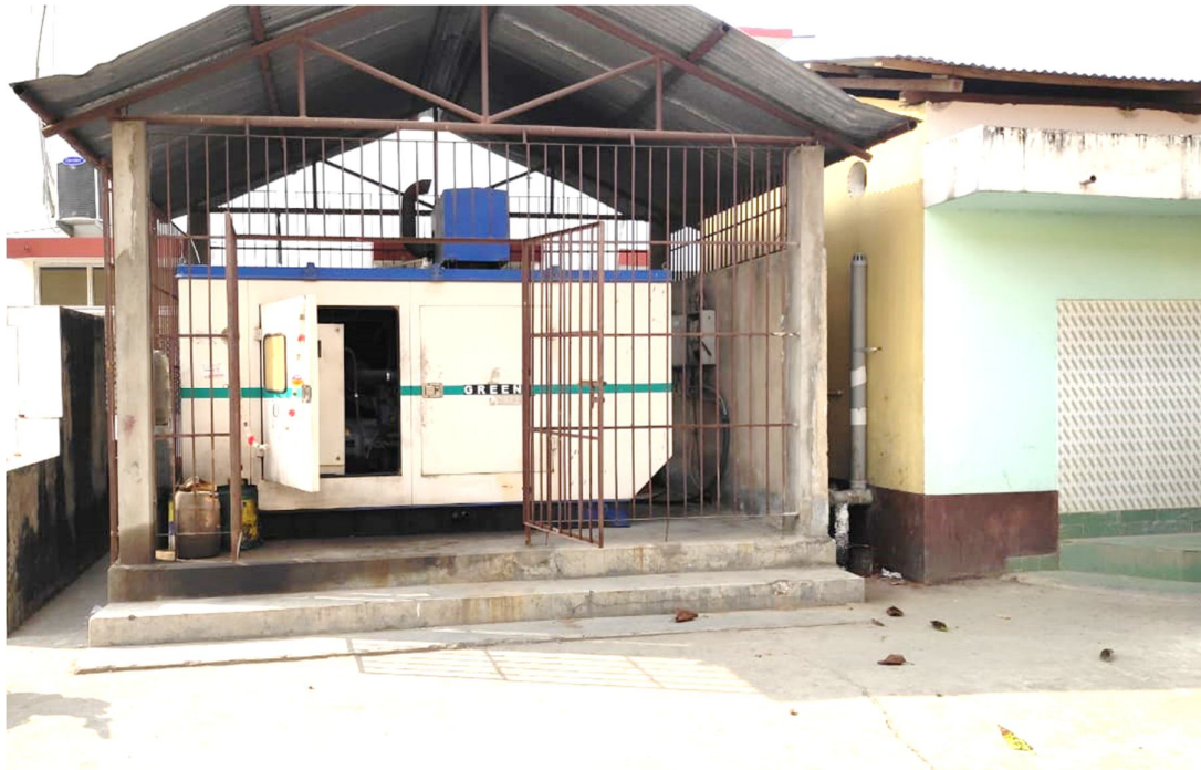
Figure 9 Diesel Generator Set
