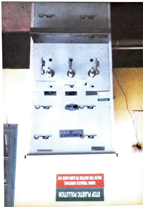
Newly set up of Drinking water facility (F-Block and G-block)
