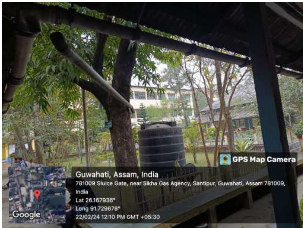
RAIN WATER HARVESTING FACILITY
