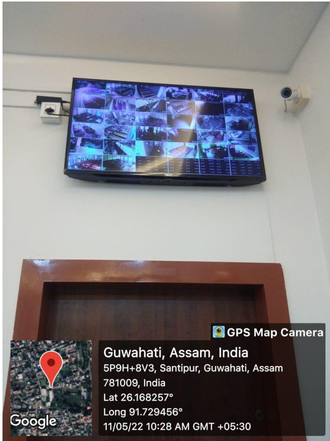
CCTV cameras for digital monitoring.
